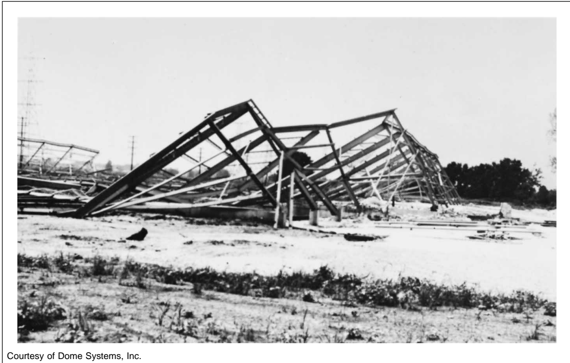
Fig. 3. Wind damage to steel frame. This framework is only one of many that did not have adequate cable bracing.
